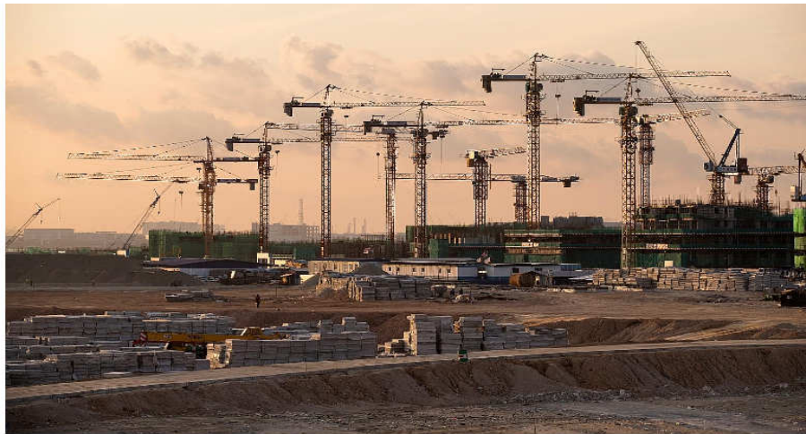
Cranes at the Forest City project in Johor. Malaysia's construction firms have seen great growth in the number of projects to execute, but there remains a concern over the glut in the property market. PHOTO: BLOOMBERG
